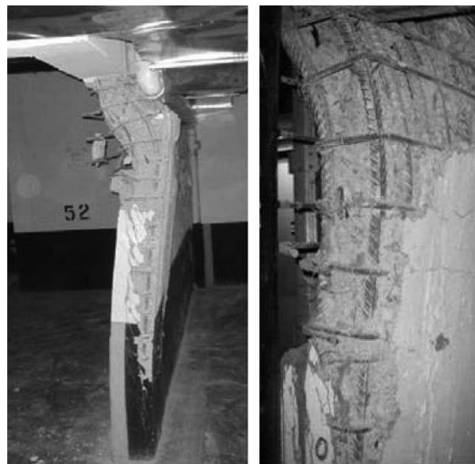
Figure 10. Boundary Crushing and Reinforcement Buckling Failure [2]
