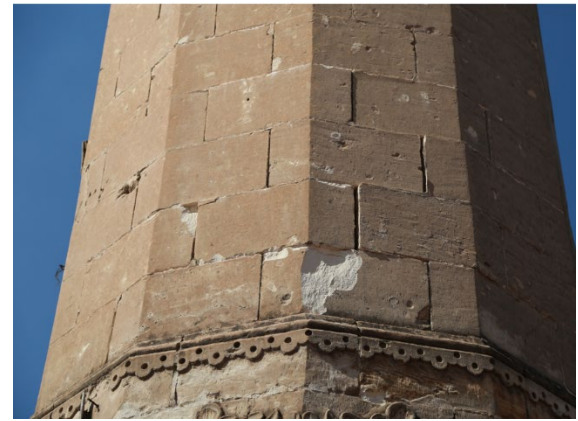
Figure 2. Crushing in the minaret pedestal and body stones, joint separations
