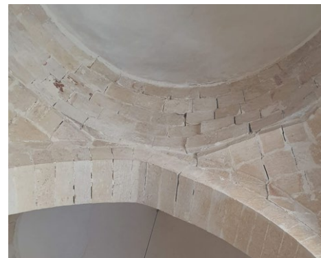
Figure 4. Carrier arch damage
